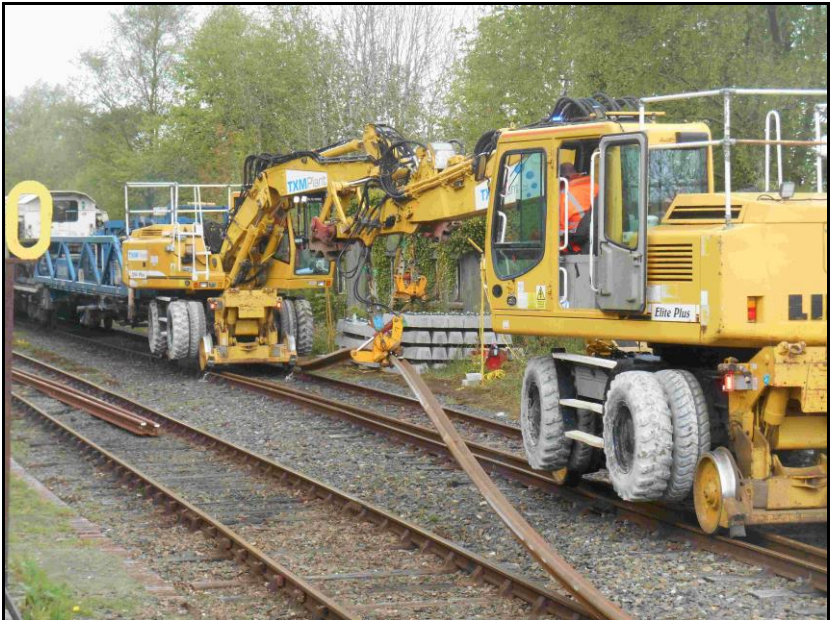
Lifting continuous welded rail off formation ahead of the track laying machine.
